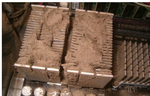
Figure 11. Heatsink inside electronic enclosure exhibiting extreme dust accumulation.
